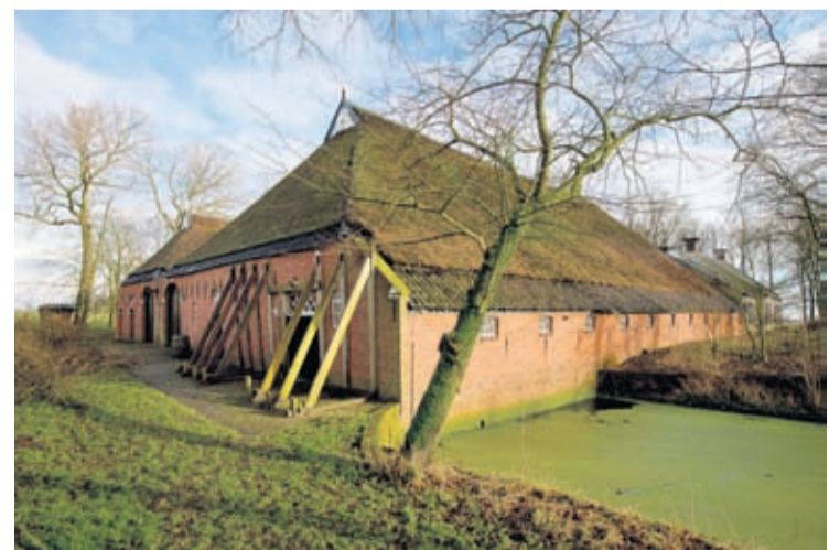
Support beams stabilize an historic farm after a series of small tremors caused by decades of gas extraction, in Hunzinge, in Groningen province, northern Netherlands on Jan. 19, 2018.
